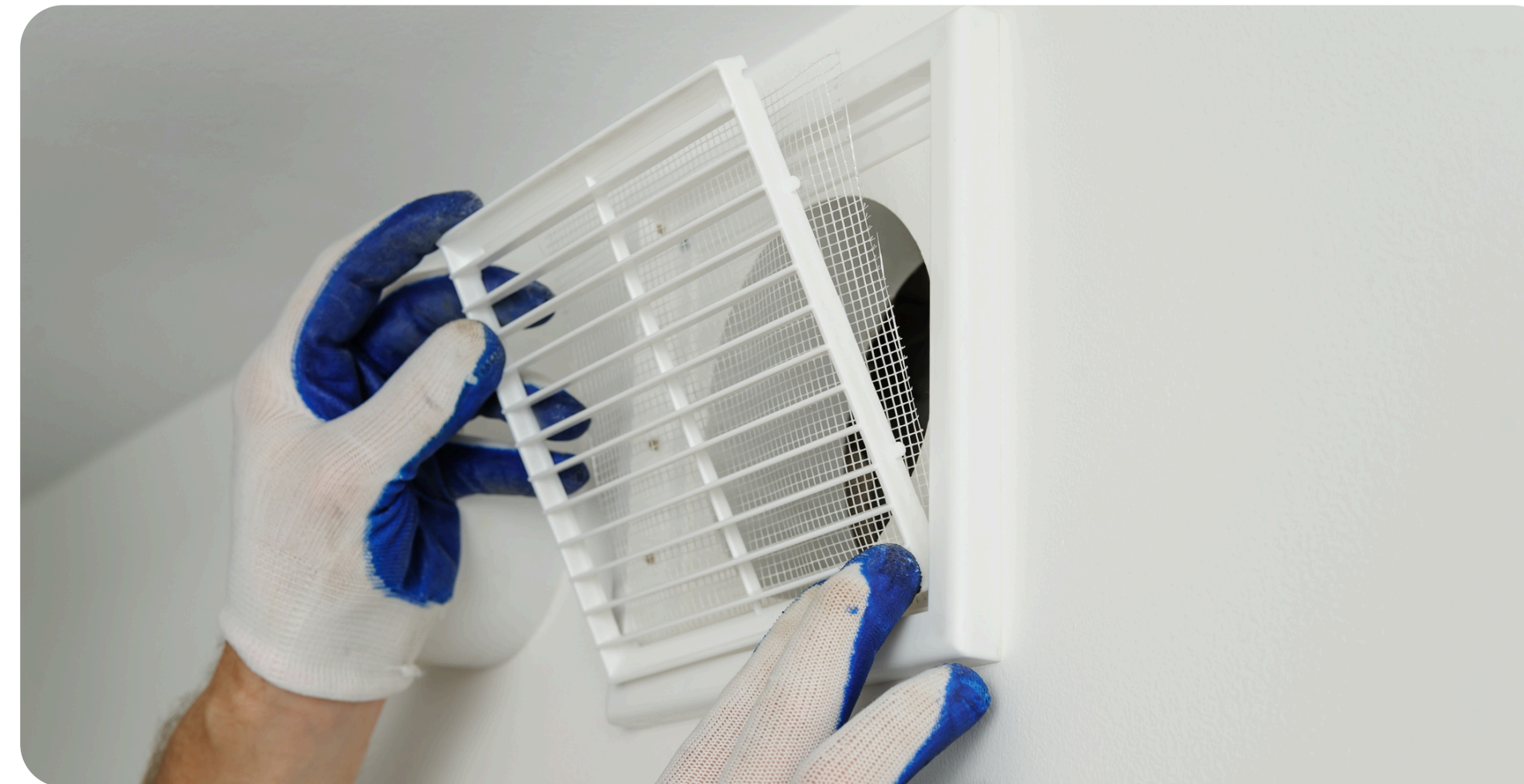
Ventilation installation in a home. Credit: Canva stock image
